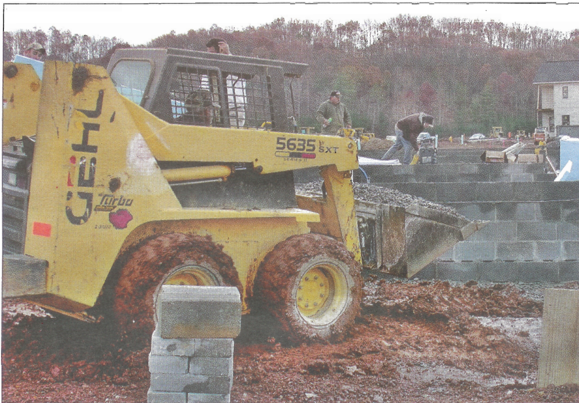
Workers with Christopolous & Kennedy General Contractors lay foundations for townhouses at Grove Parks Commons, which recently won an award from the American Planning Association's Tennessee chapter for Outstanding Green Community.
