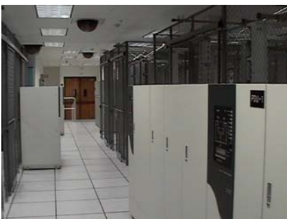
Santa Clara Network operations center
